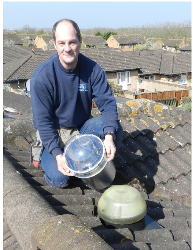
A Solarspot installer compares our acrylic dome with a 4 year old Solatube dome.
