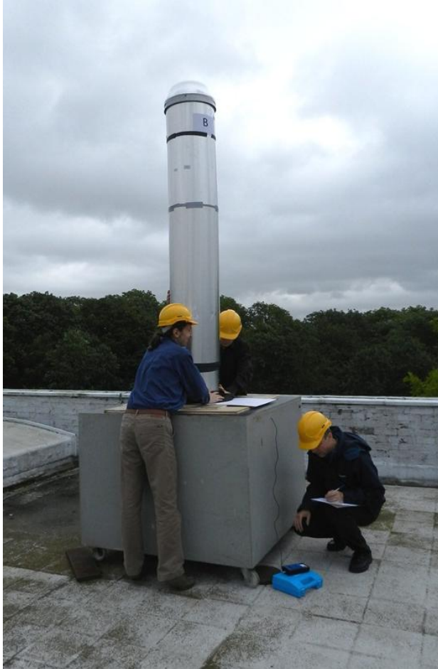
Figure 4 Light tube (Solarspot D-38, single glazed top dome, no Convax lens) under test on roof
